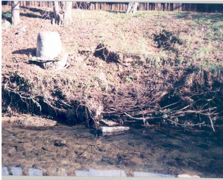
Figure 3.3. Erosion in the upper part of the Cumberland segment. Top : Looking upstream towards the Cumberland Avenue box culvert. Bottom : The left bank of the stream between two footbridges. A tree was undermined and fell into the stream at this location. (Photographs by the author.)
