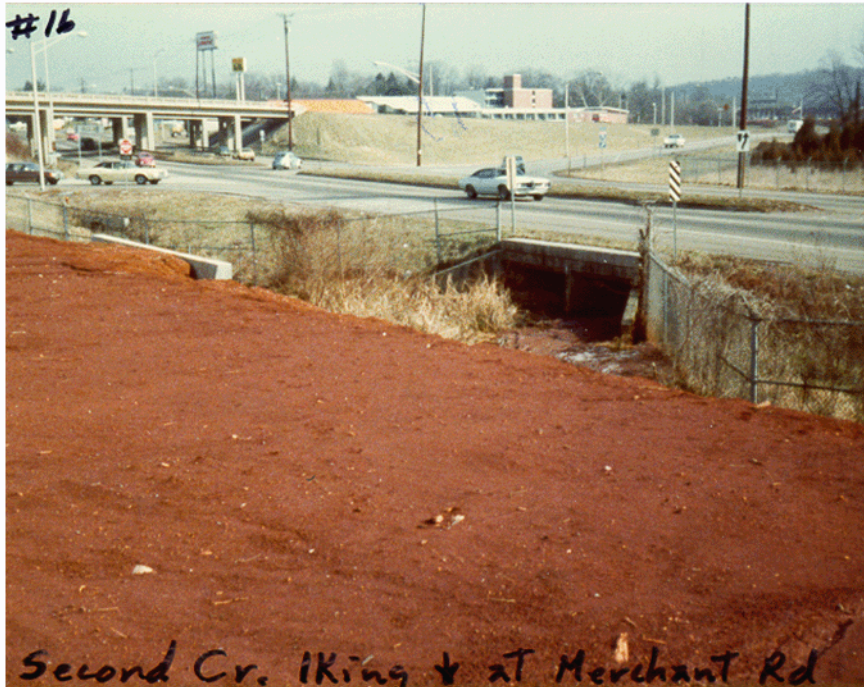
Figure 3.25. Bare soil exposed during construction projects. Top : Looking south towards the I-75 – I-640 interchange. Bottom : Looking south at Merchant Drive. Both photographs were taken in 1979. (Photographs from TVA archives, Knoxville, TN.)
