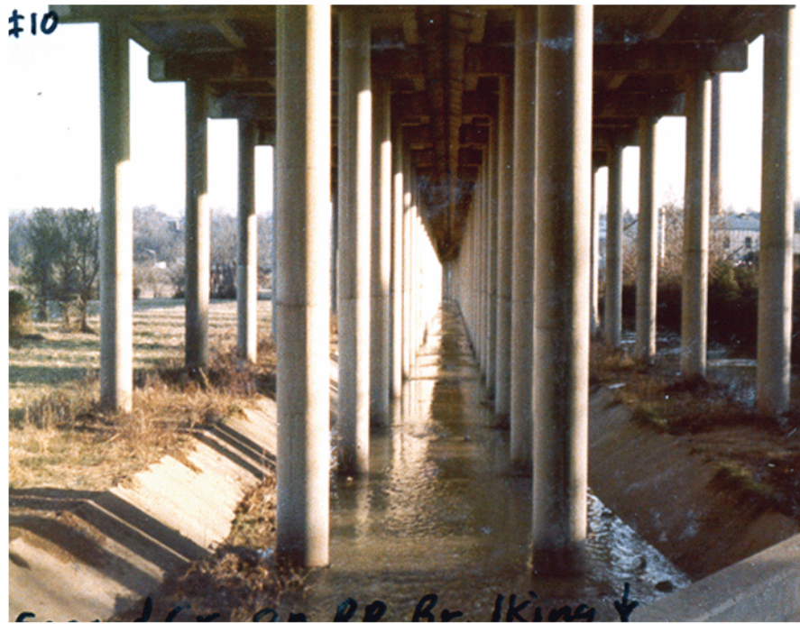
Figure 3.27. Support piers for I-275 in Second Creek in 1979. The view is upstream in the top photograph and downstream in the lower one. (Photographs from TVA archives, Knoxville, TN.)
