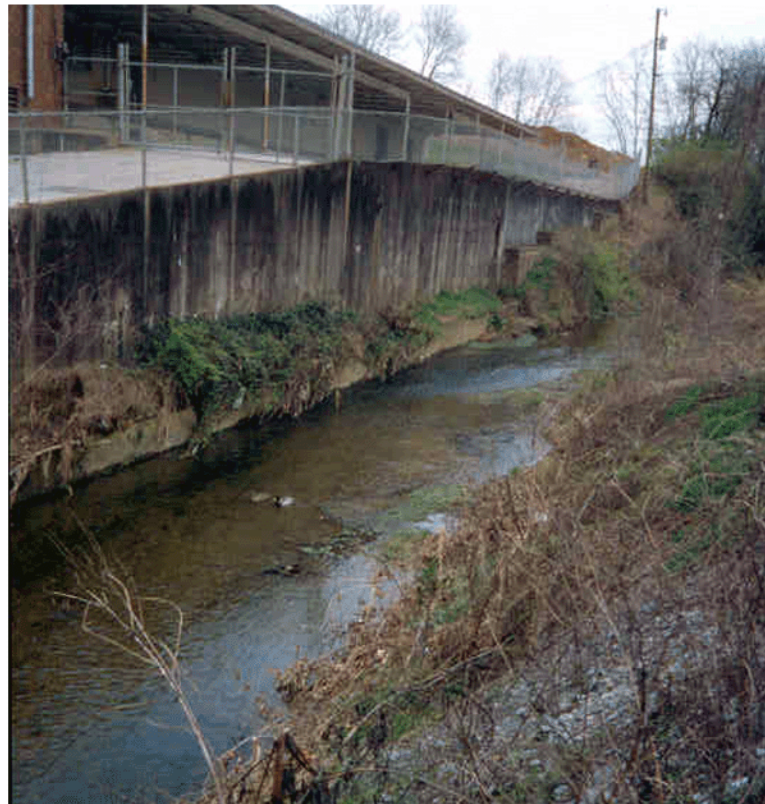
Figure 3.6. Rock and concrete walls downstream and upstream of Bernard Avenue. Top : Looking downstream from close to Bernard Avenue. A railroad bridge can be seen at the right side of the picture. Bottom : Looking upstream. (Photographs by the author.)
