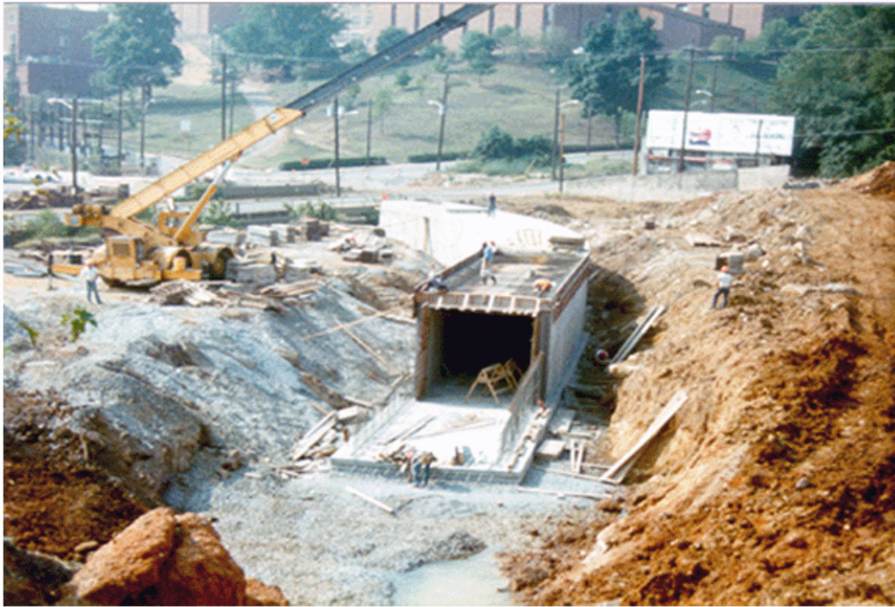
Figure 2.18. Construction in the channel of Second Creek upstream of Cumberland Avenue. These photographs were taken in 1980. (Photographs from TVA Archives, Knoxville, TN.)
