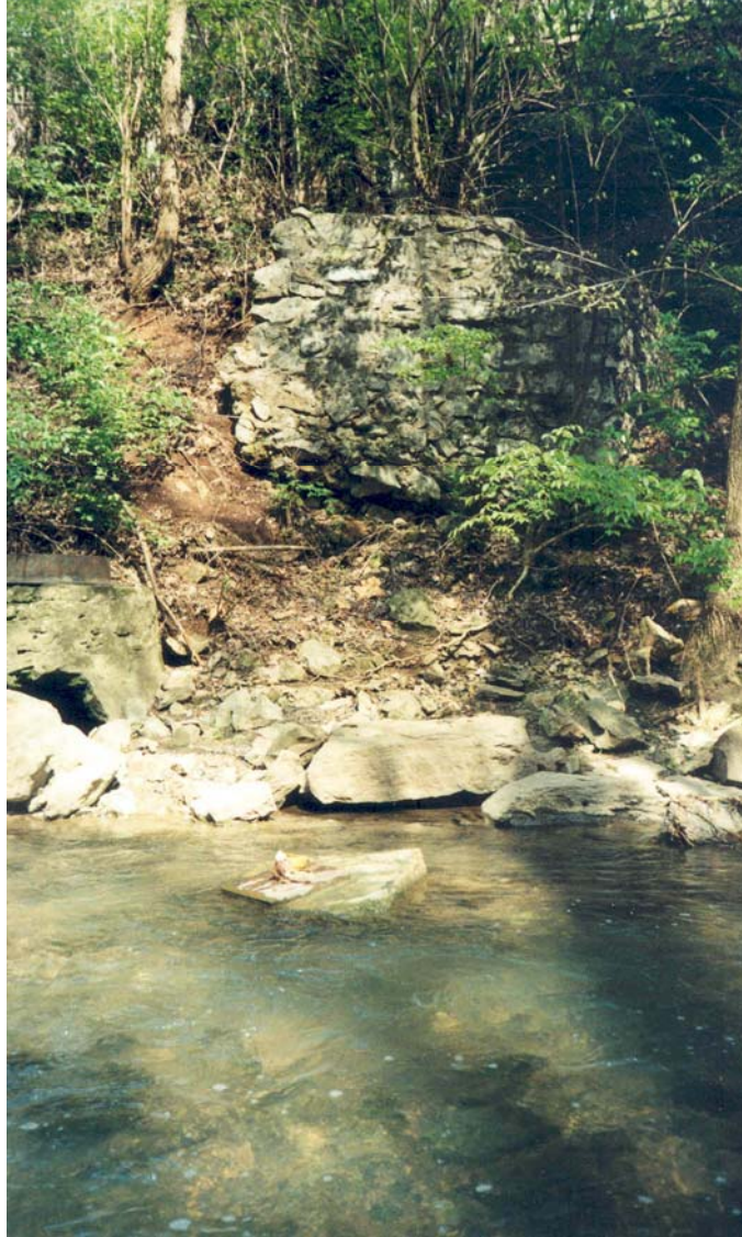
Figure 3.4. Part of an old wall poised to slide into the stream. This location is between sites U and UT on the east side of lower Second Creek. Large rocks at the base of the banks, as seen here, are common in this segment of the stream. The water flows from left to right in the picture. (Photograph by the author.)
