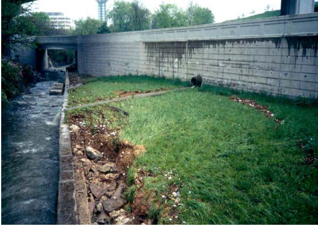
Figure 3.5. The channel near Western Avenue. The channel banks along this part of the stream are lined with concrete, shaped rock, or riprap. This view is looking downstream. World's Fair Park Drive crosses Second Creek in the upper left part of the picture. (Photograph by the author.)
