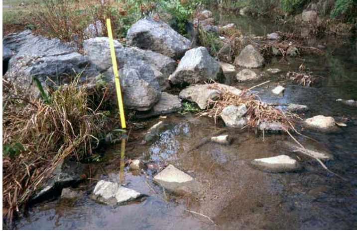
Figure 3.17. Large rocks placed near the Inskip Avenue Bridge. View is looking upstream. The yellow bar is 1.22 m (4 ft) long. (Photograph by the author.)
