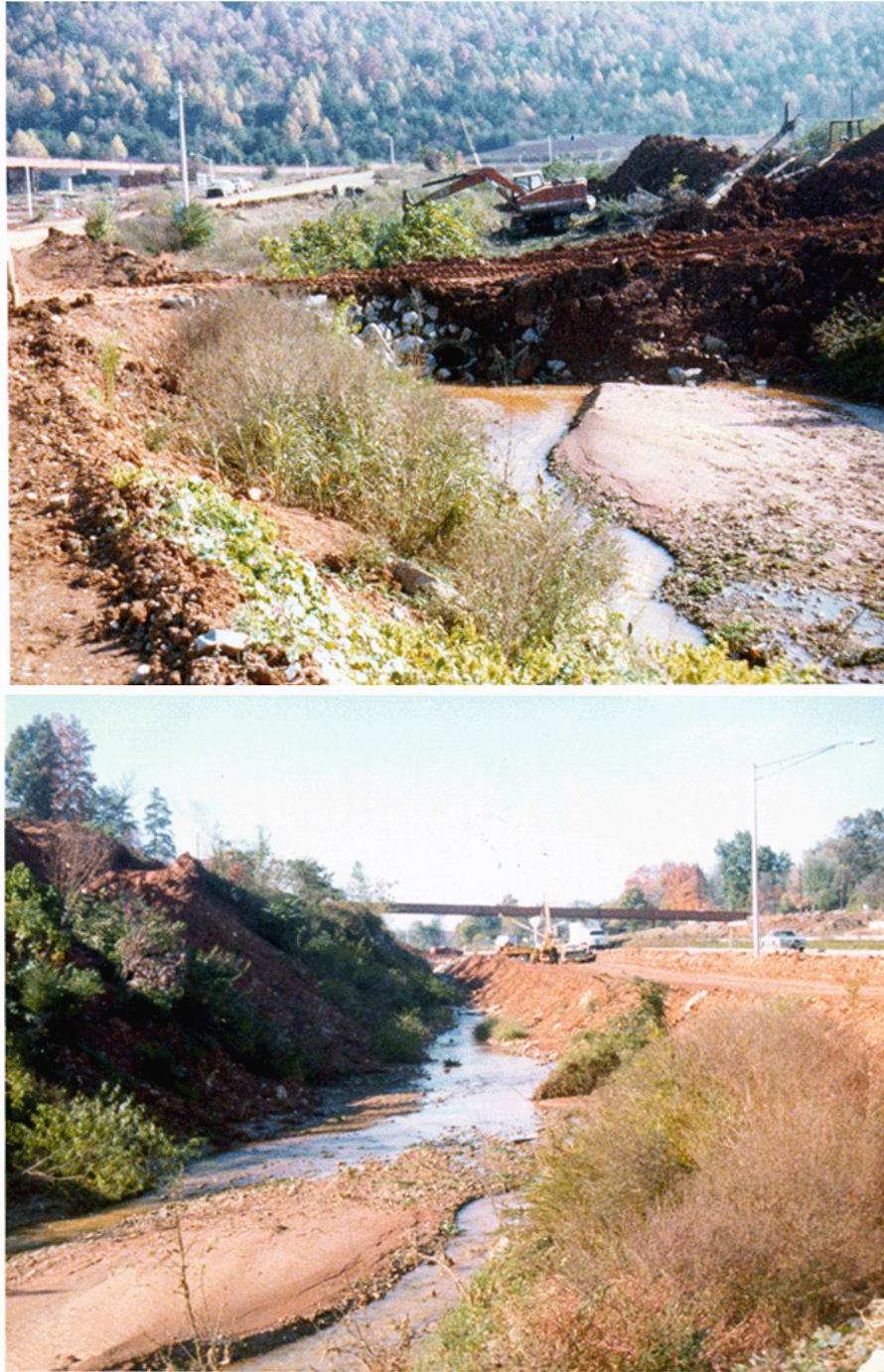
Figure 5.7. Sediment in the channel during construction in 1979. This location is upstream of the I-75/I-640 interchange and Sharp Ridge. The Tillery Road overpass is visible in the background. Photographs courtesy of TVA.
