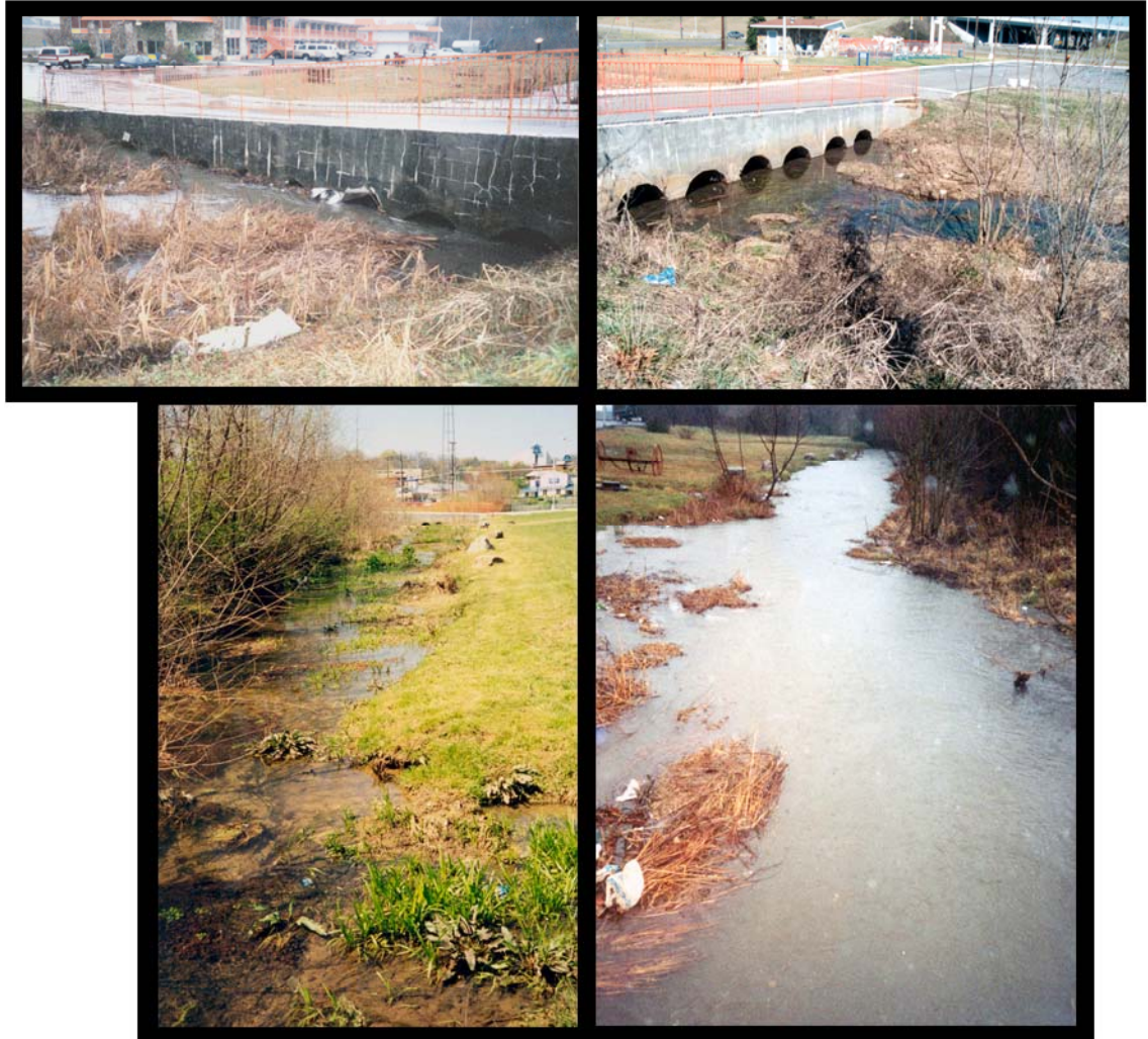
Figure 3.21. Second Creek near the Motel Bridge. Top left: The upstream side of the Motel Bridge during a modest high water event. Some debris was collecting at the culvert entrances. A stain above the top of the culverts reveals the level of a recent flow. Top right: The downstream side of the Motel Bridge, at a time of low flow. Bottom left: Looking upstream towards the Motel Bridge. The left bank is in grass, but the right bank contains thick shrubs and trees. Sediment in the channel at this location is almost knee-deep. Bottom right: Looking downstream from the Motel Bridge during the same runoff event as shown in the photograph in the upper left. The channel narrows considerably about 5 m downstream from the bridge. (Photographs by the author.)
