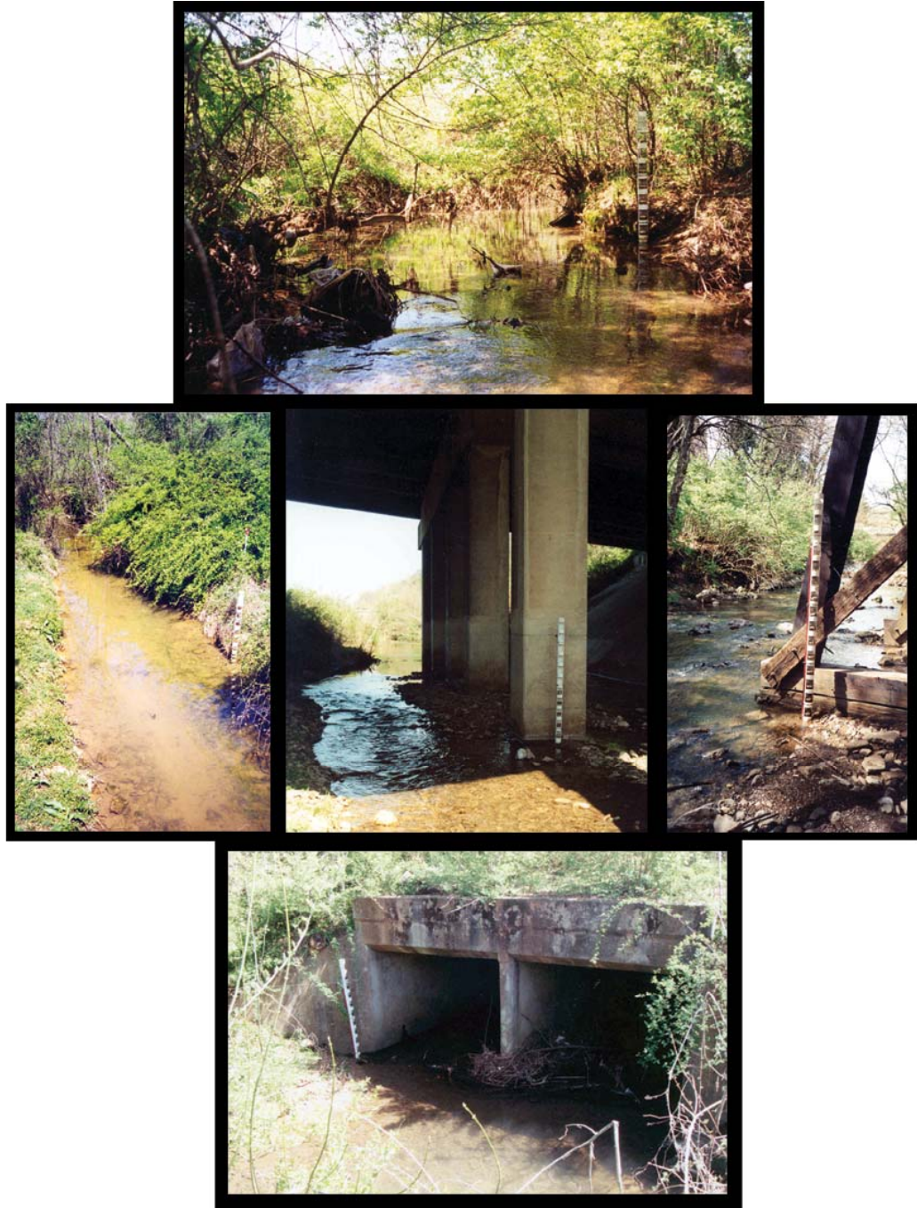
Figure 4.4. Photographs of rising stage sediment samplers in place. Top : The Inskip site sampler, looking upstream. Center left : The sampler is in the right side of this photograph of the Dutch Valley Tributary, looking upstream. Middle : The Heiskell location, looking upstream. The shadow of the farthest downstream support can be seen at the base of the sampler. Center right : Sampling site U, looking upstream. Bottom : Site C, looking downstream. (Photographs by the author.)
