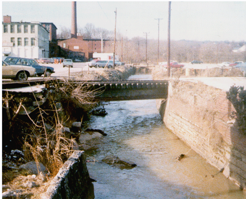
Figure 3.8. Brick and concrete walls upstream from Baxter Avenue. Even in 1979, at the time of these photographs, parts of the walls were falling into the creek. More damage had occurred by 2001. Top : Looking downstream at the culvert under Baxter Avenue. Bottom : Looking upstream from Baxter Avenue. (Photographs by the author.)
