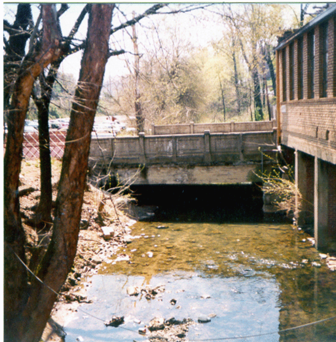
Figure 2.17. Second Creek upstream of Cumberland Avenue in 1979. This part of the creek now flows underground in a large box culvert. Top : looking upstream. Bottom : looking downstream. (Photographs from TVA Archives, Knoxville, TN.)
