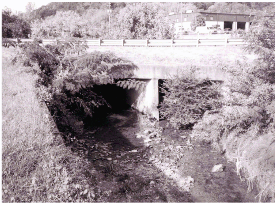
Figure 3.26. Old and modern photographs of the Heiskell culvert area. The triple box culvert shown is located under the on-ramp to I-275 N. Top photograph was taken in 1979, the lower photograph in 2001. (Top photograph from TVA archives, Knoxville, TN. Bottom photograph by the author.)
