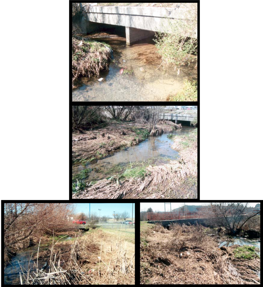
Figure 3.19. The channel close to Merchant Drive. Top : The downstream side of the culverts under Merchant Drive. Low flow is diverted toward the viewer by the accumulation of sediment in the center left of the photograph. Middle : Looking at the culverts from farther downstream. View is from the left bank. Bottom left : Looking upstream towards Merchant Drive. There is a great deal of vegetation on the sediment in the channel. Bottom right : Looking downstream along the left bank. One culvert under the Motel Bridge is visible to the right of the tree. These photographs were taken in 2000. The trees were cut down less than a year later. (Photographs by the author.)
