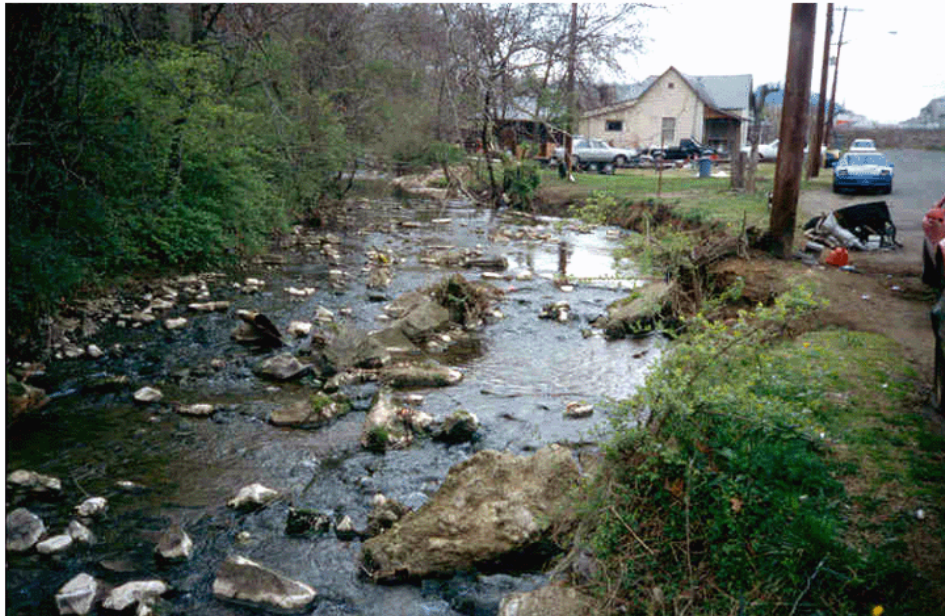
Figure 3.9. Severe erosion upstream of the Oldham Avenue Bridge. The eroding streambank threatens a utility pole and part of Davanna Street. Top : Looking toward Davanna Street. Bottom : Looking upstream. Devanna Street is visible on the right. (Photographs by the author.)
